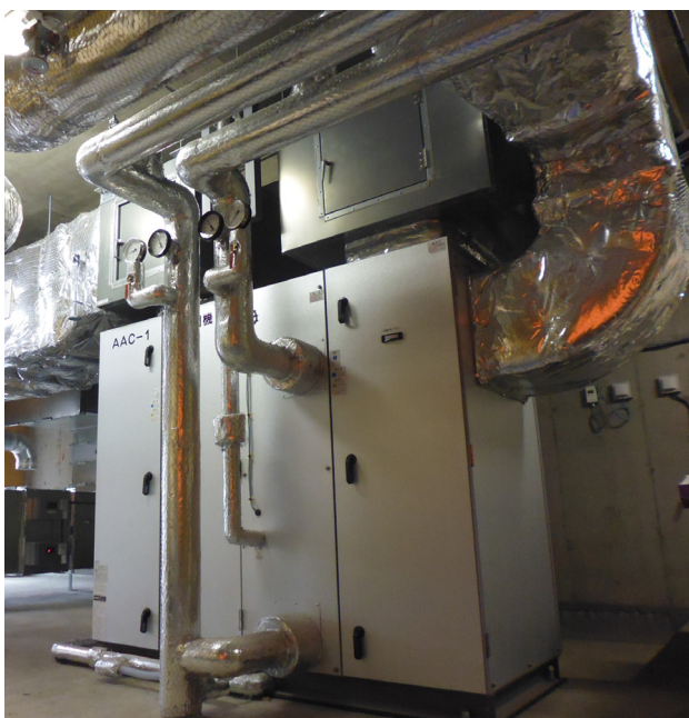
An experimental facility for HVAC systems, showing an air handling unit undergoing testing. Source: Building Research Institute, Japan
